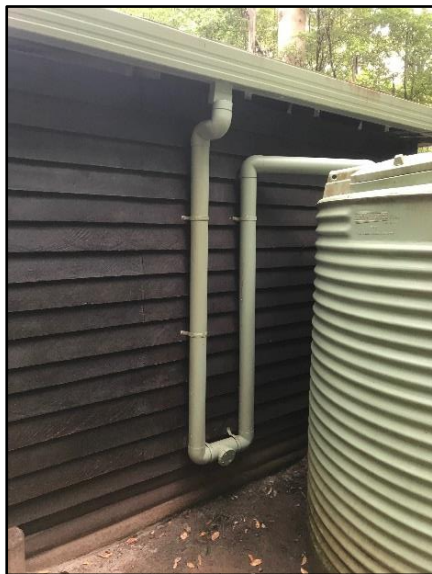
U-shaped pipe with drain cap
